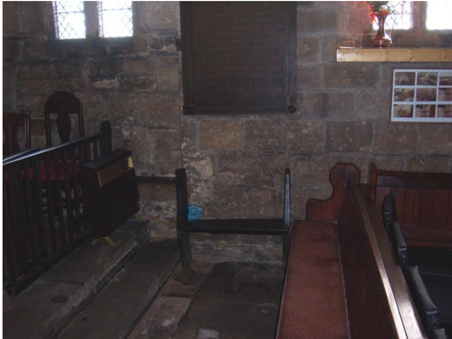
Figure 36 View west into chancel. Pews, altar rail and commemorative board are all visible
