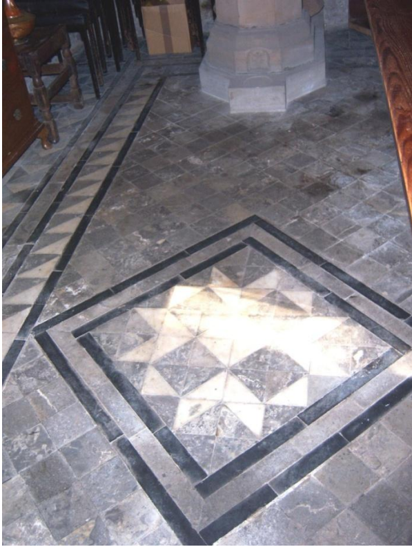
Figure 28 Marble and slate tiled floor in a geometric pattern in the Unsworth Chapel
