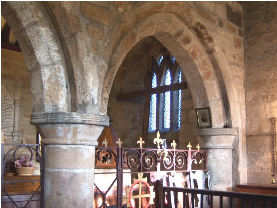
Figure 33 View north east into Unsworth Chapel showing two of the three columns of the arcade which separates the Chapel from the chancel
