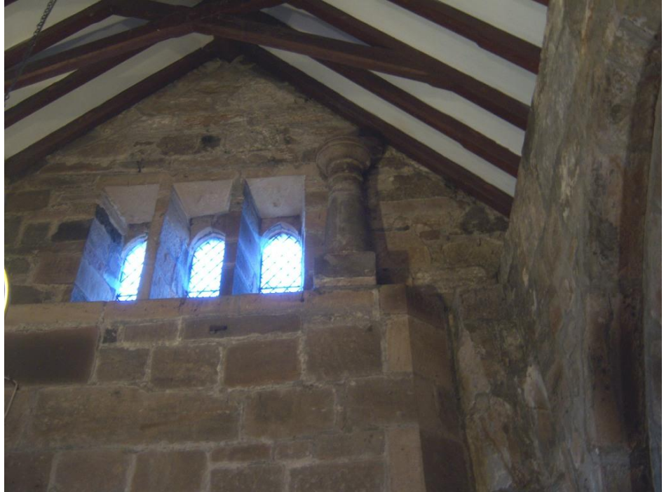
Figure 42 Small pillar like object on window ledge of chancel west wall. Believed to be former sundial shaft
