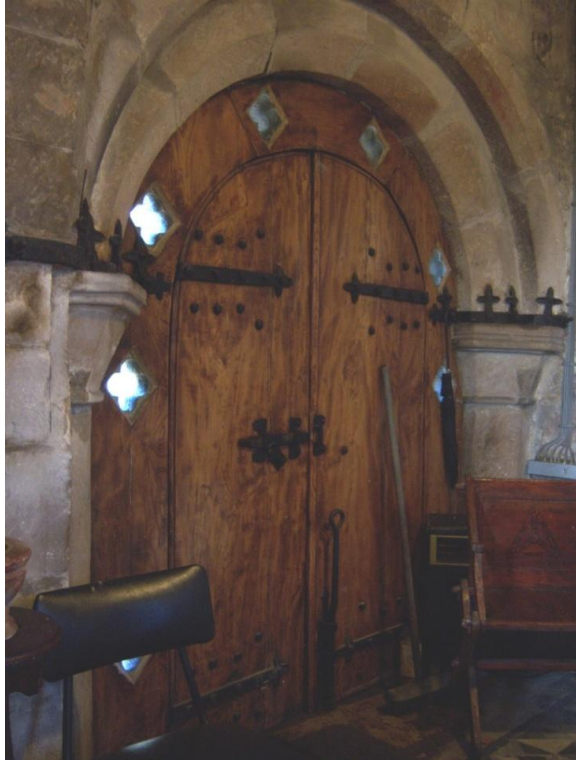
Figure 26 Oak entry door with decorative cast iron strap hinges and quatrefoil window detailing
