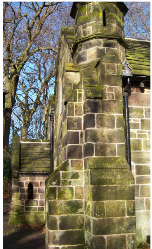
Figure 19 Angled buttressing at south west corner below the bellcote
