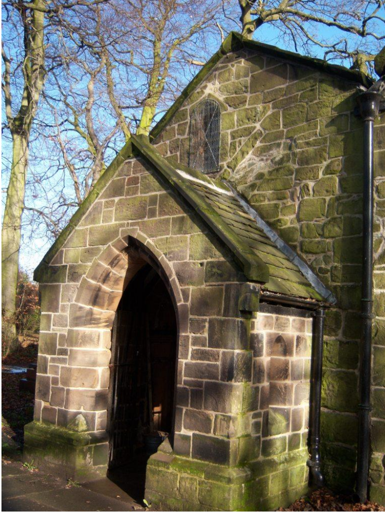
Figure 17 Western elevation and porch entrance – a former roof line is visible at an angle immediately below the lancet window
