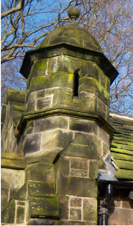
Figure 18 Bellcote on south west corner – dating from 1775 but moved into present position during 1830s changes
